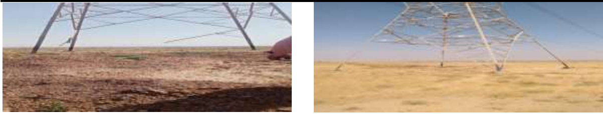
Figure 4: Theft of materials in fragile locations, weak structures collapse with climatic impacts
